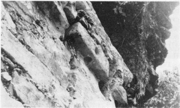
Fig. 2 Palenque. Holes of the vault spring: (a) holes in the medial support wall, Temple of the Sun; (b) detail of holes, Temple of the Cross.
